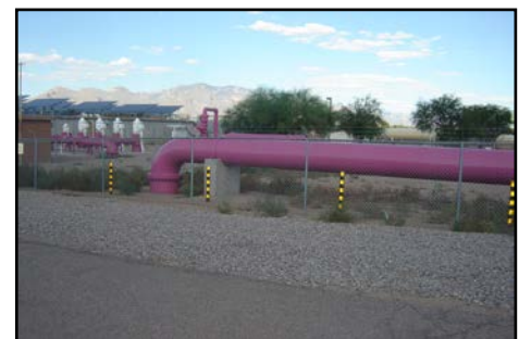
Purple irrigation pipes for treated effluent
