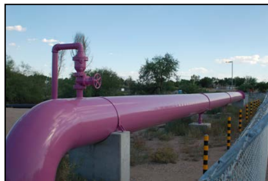
Reclaimed water distribution line
