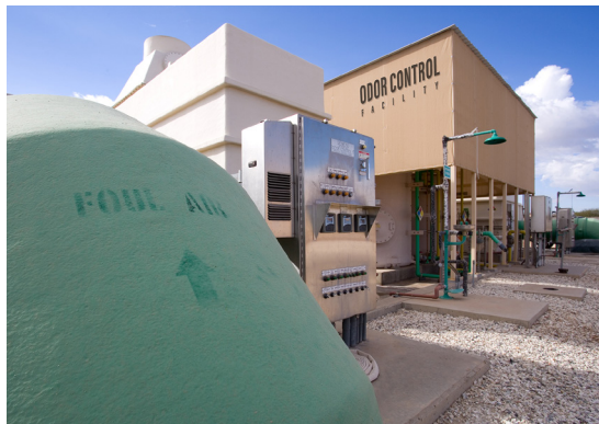
State-of-the-art Odor Control technology effectively controls odor throughout the facility.
