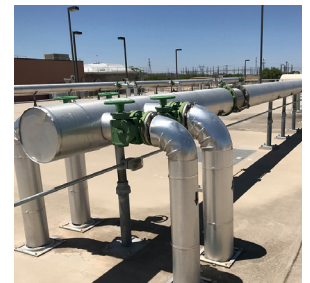
Aeration Facility where oxygen is forced into the waste stream creates microorganisms that break down wastewater contaminants.
